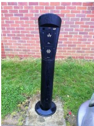
Example of an electric vehicle recharging point.
