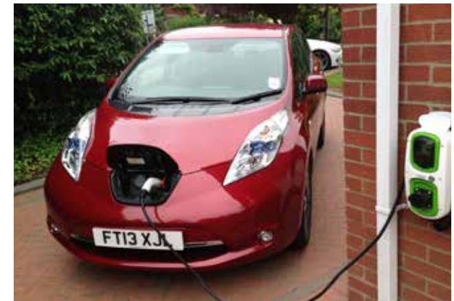
Figure 186: Off-street mounted car charging points
